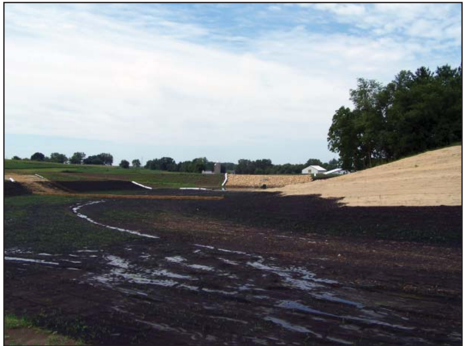
The 30th Street project was still under construction during the summer of 2008. This large retention basin drains 200 acres of land within the city of Monroe, Wisconsin. Photo: Barbara Ellis - FEMA
