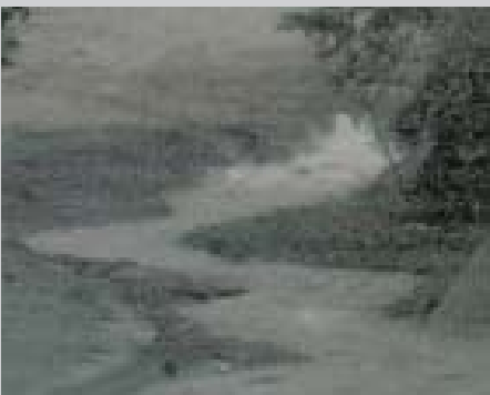
Water boils out of an inlet culvert in the half-finished 30th Street Project during the June 2007 floods in Monroe.
