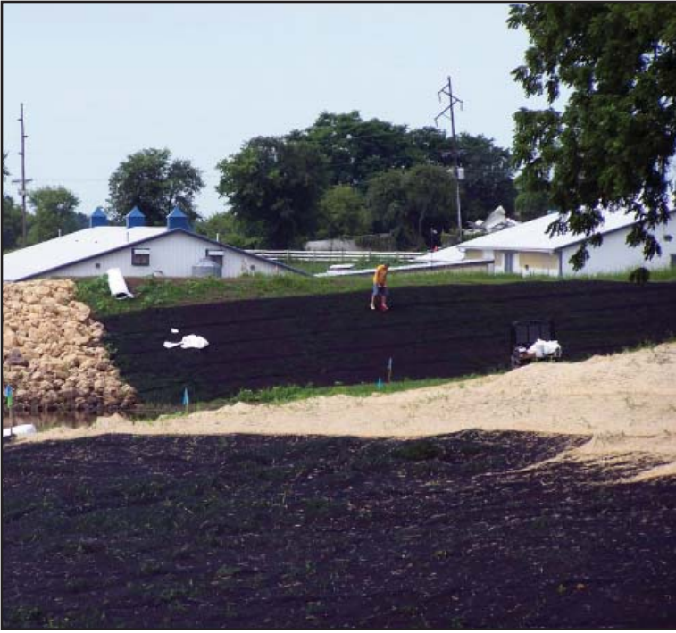
A worker staples down plastic erosion control mat that stabilizes sloping sides of the 30th Street retention basin.
